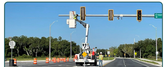
Installation of traffic sign at westbound 44th Avenue East and Creekwood Boulevard
